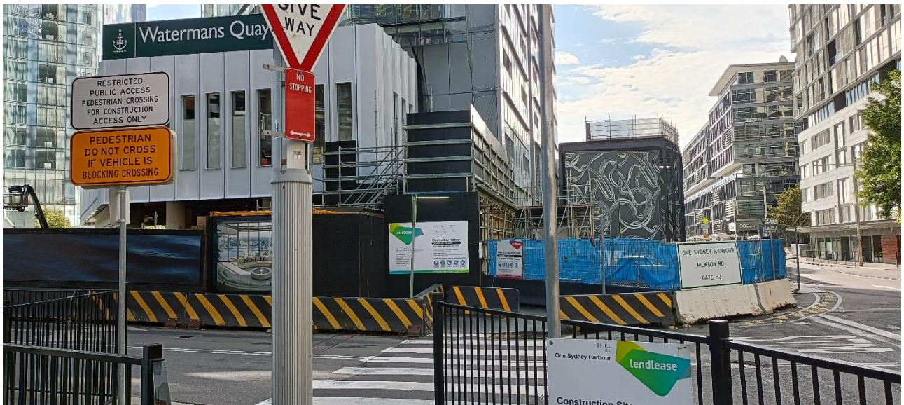
Photograph B.2 Waterman Quay Rd looking North showing main access gate layout and road interface.
