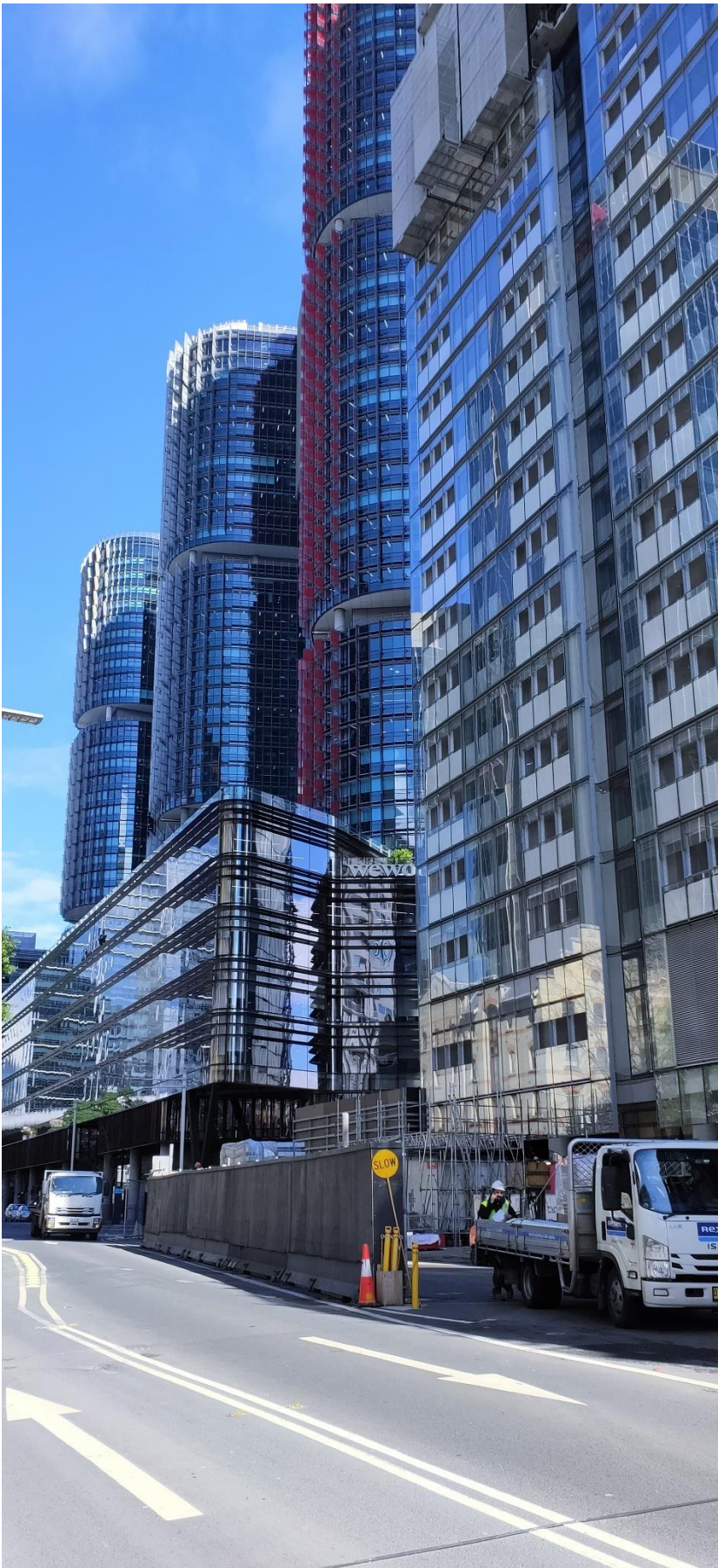
Photograph B.8 View of Gate H3 on Hickson Road showing façade treatment progress.
