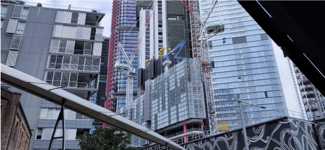
Photograph 4: External – Hickson Road looking South showing both cranes and active concrete pour.
