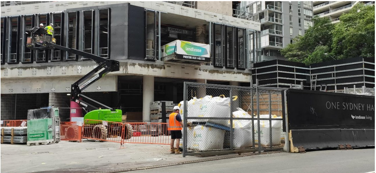
Photograph B.2 Waterman Quay Rd looking North showing main access gate layout and road interface.
